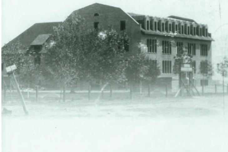
The 1935 earthquake also rendered unusable the Deaconess School's new building, the nearly completed Van Orsdel Hall, on the right in this photograph of the campus. The building still stands today, a lonely shell in the Prickly Pear Valley.
