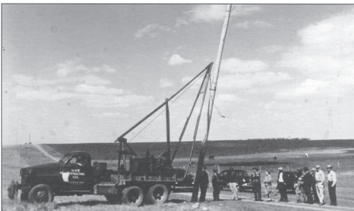
Anna Boe Dahl and other members of the Sheridan Electric Co-op board of trustees watch as one of the first poles is erected in Sheridan County in 1947.
